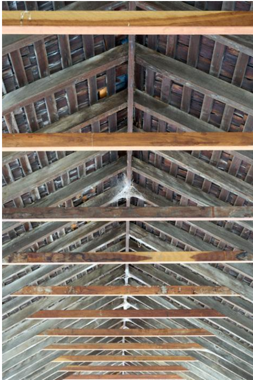
Detail of the roof of the laundry area, with the original wooden shingles showing
